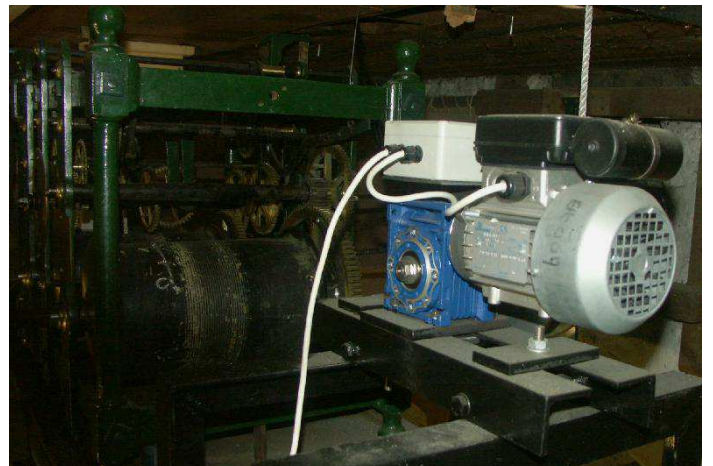
Auto-winder installed in 2005
